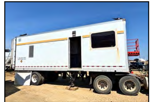
2007 Manac, new electrical, console and pug box, 200 HP soft start, (1) VFD, 12 starters
