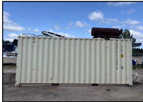
20 ft sea can with 2012 Cummins QSK23 600 KW prime power gen set, 0 hrs on fresh rebuild. main breaker
