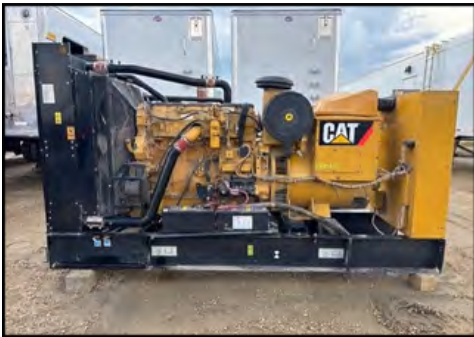
2008 Cat C15 410 KW prime power uni 7,654 on fresh rebuild
